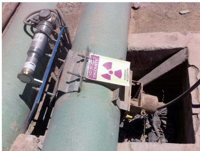
Figure 4: Installation with new detector and old source
