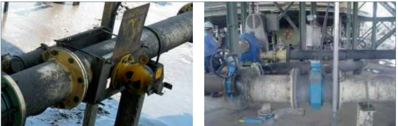
Figure 2: b) Thickener application – real installation
