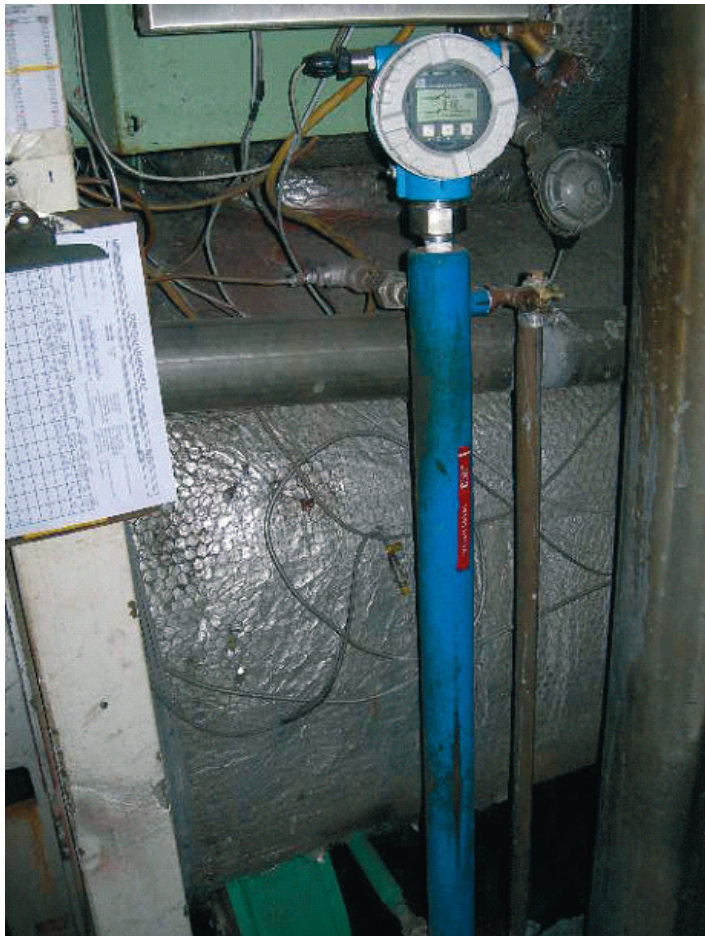
Levelflex M FMP40 installation in canned soup production
