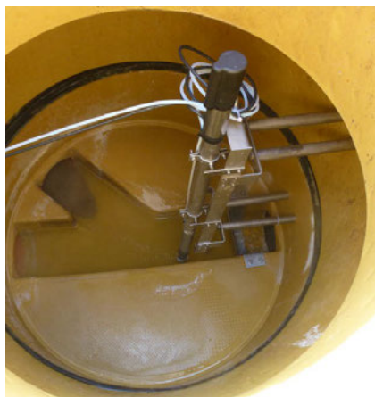
The Memosens sensor Viomax CAS51D is installed in a sewage shaft for the monitoring of COD in dairy effluent.
