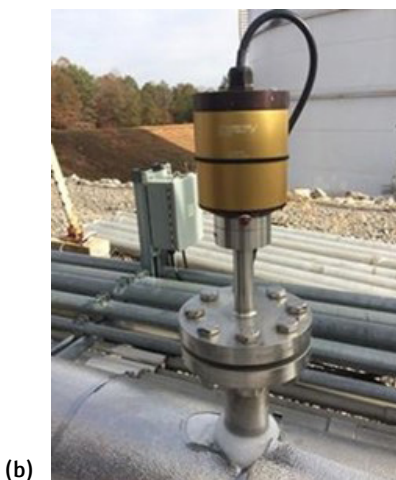
Figure 4: Typical installations of the Rxn-41 probe on LNG transfer lines between the storage tank and truck loading area at (a) the first site, a peak shaving LNG facility, and at (b) the second site, a satellite LNG facility.
