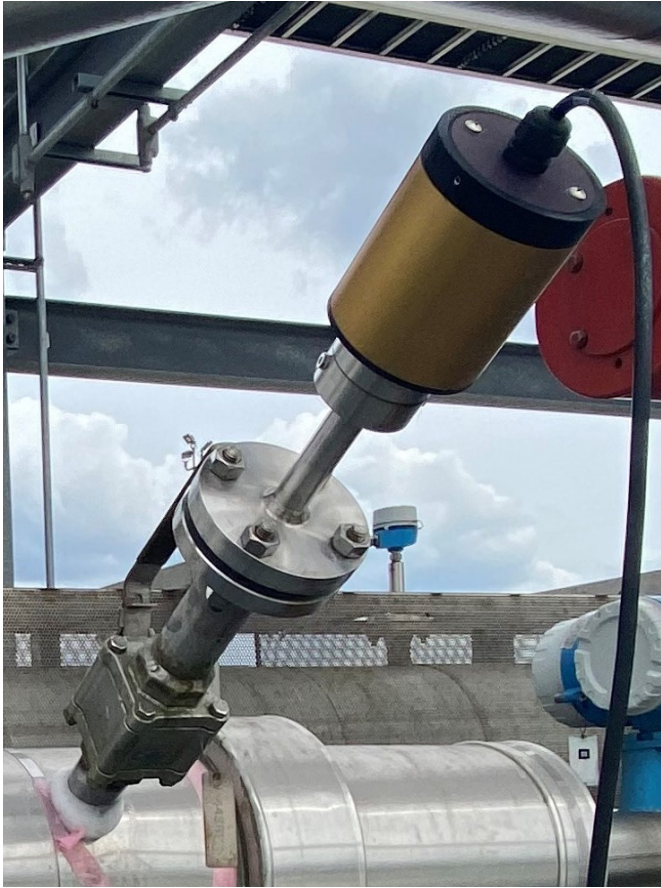
Figure 3. An Rxn-41 probe installed on an LNG transfer line similar to the one at the Fluxys LNG terminal.
