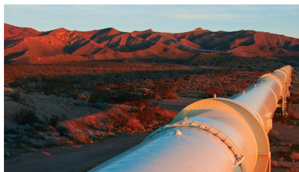
Pipelines de transport
