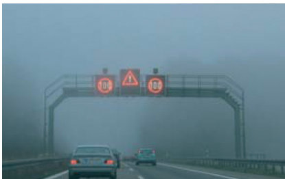
Traffic management systems
