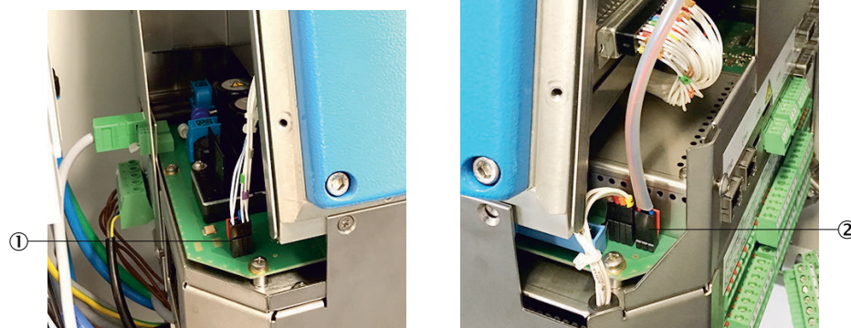
Figure 101: Pressure control module and fan lines
