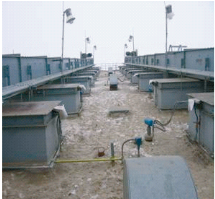
Installations in soybean extraction plant
