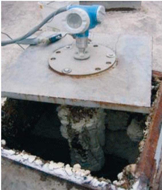
FMR250 with 4" horn installed in soybean extraction plant
