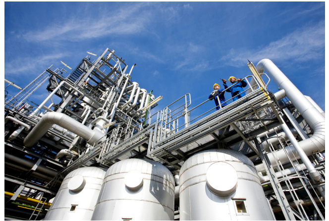
A wide variety of challenges in hydrogen production require flexible measuring devices.
