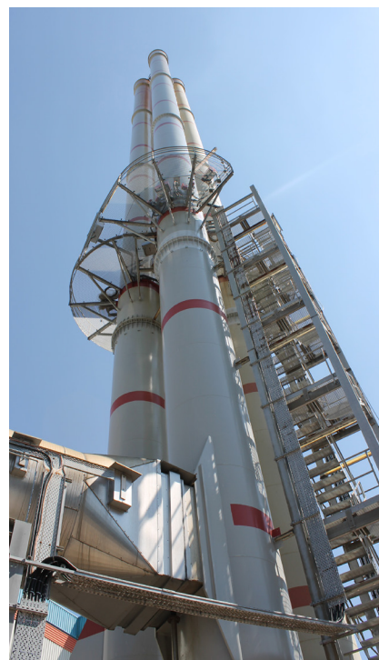
Monitoring chimney stack emissions
