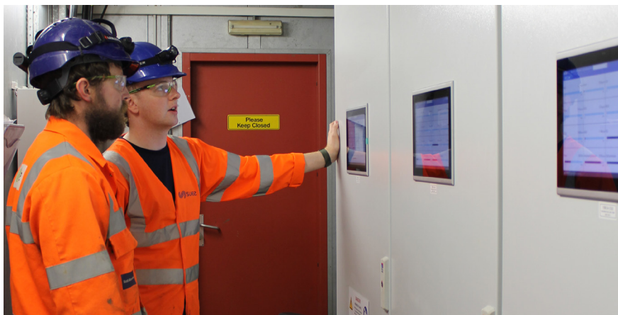
EC&I Engineer Scott Almandares and E&I Maintenance Technician Joe Wilson with the MCS200
