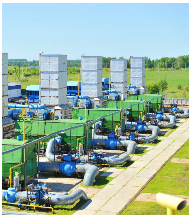
Figure 2: Example of a natural gas compression station
