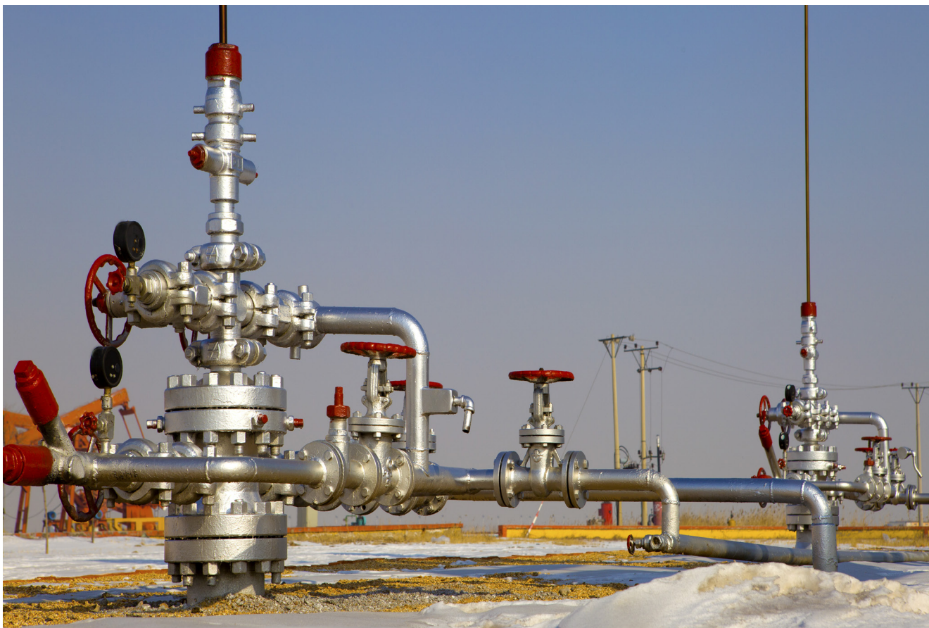
Figure 1: Example of a typical natural gas well (one of dozens in a typical storage field)
