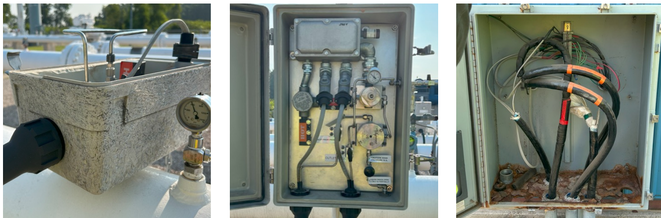
Figure 3: (Left) Heated sampling probe; (Center) pressure-reduction system; (Right) sample-distribution enclosure mounted outside the analyzer shed
