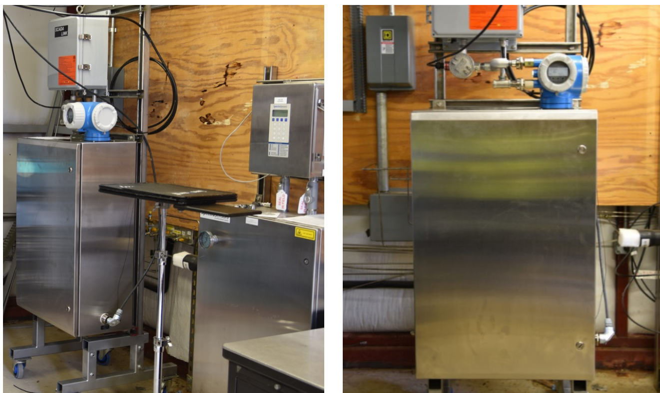
Figure 4: (Left) The Endress+Hauser JT33 TDLAS \text{H}_2\text{S} analyzer positioned beside the Endress+Hauser SS2100 TDLAS \text{H}_2\text{S} analyzer; (Right) front view of the JT33 TDLAS gas analyzer with a small control enclosure mounted above it
