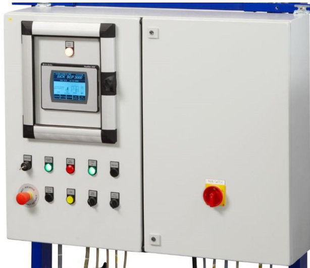
Fig. 13: Control and power supply cabinet
