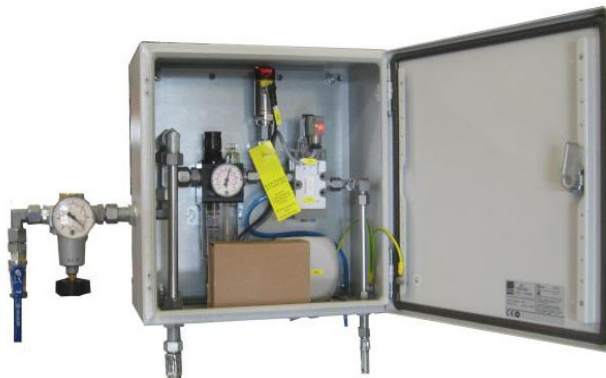
Fig. 14: Pneumatic/compressed air service unit
