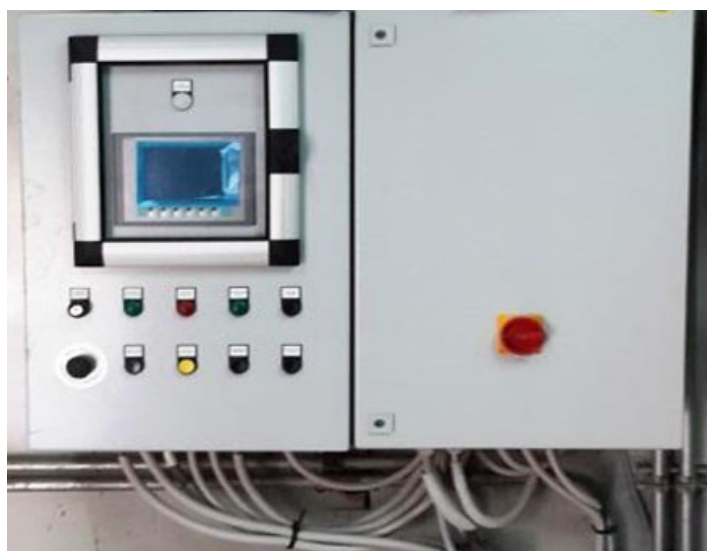
Fig. 36: Installed control cabinet
