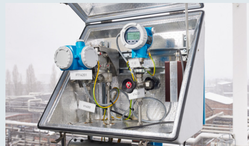
Obstruction within the impulse line
