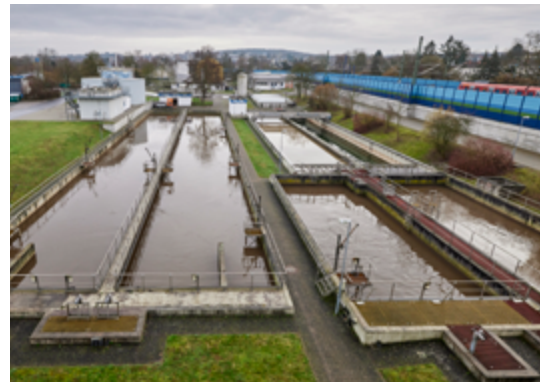
The plant handles 9,000 cubic meters of water every day.
