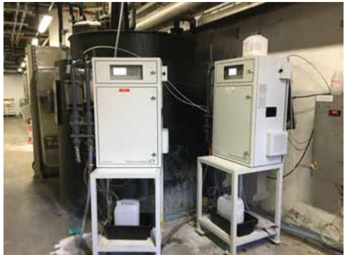
Both CA72TOC analyzers in use in outlet of biological wastewater treatment process.
