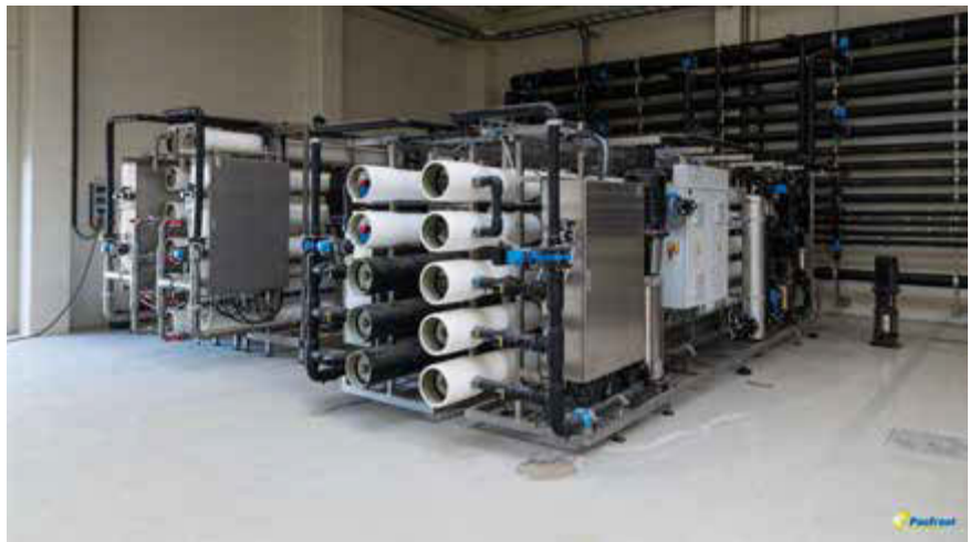
Reverse osmosis system at the Pasfrost plant.
