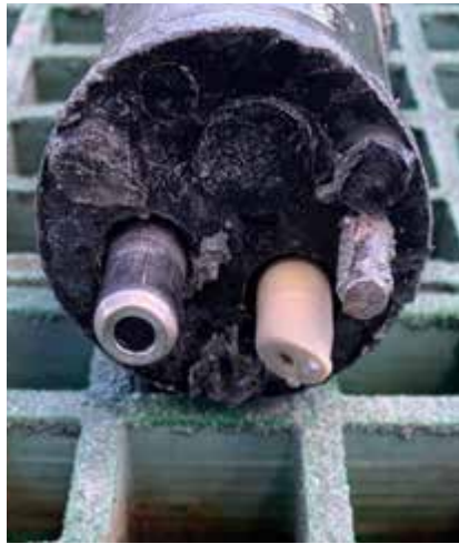
CPA111 with COS81D and CPS47D in cyanide leaching measuring point. Plastic protection stands are completely worn out but sensors are not.
