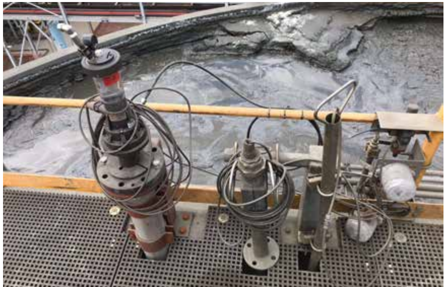
A measuring point at the leaching tank.
