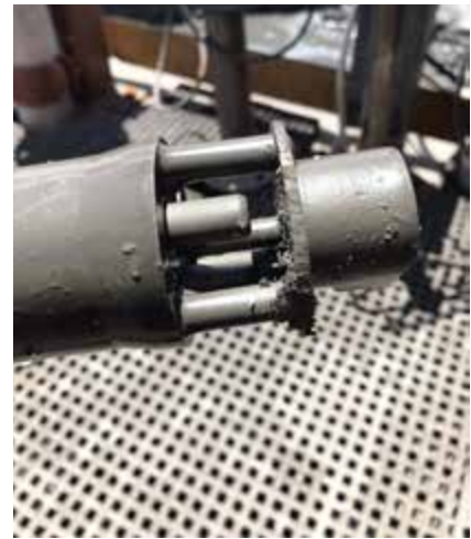
CPA111 with sensors covered with slurry, before cleaning.
