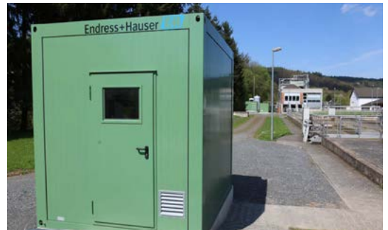
Turnkey container solution at WWTP in Breuberg-Hainstadt in Odenwald
