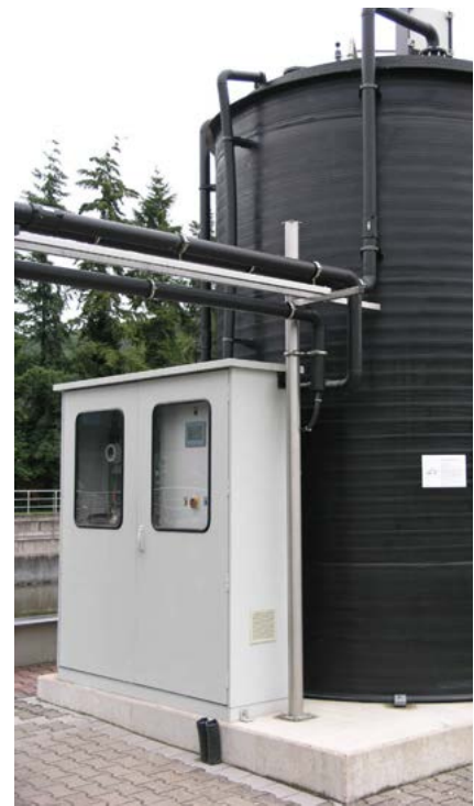
Precipitant station at Breuberg-Hainstadt WWTP (above), flowmeters for precipitant dosing (left)
