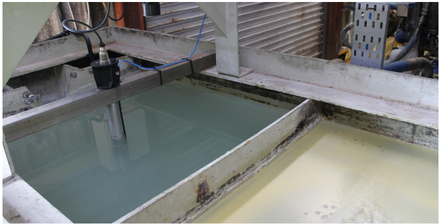
Memosens CAS80E in treated effluent tank
