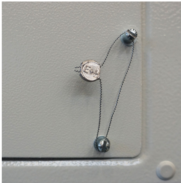
26 Screws sealed with sealing wire
