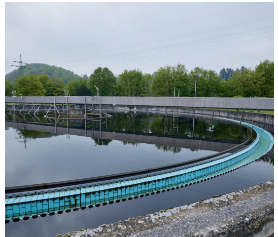
Efficient level management in sewer management
