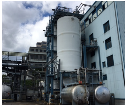
Tank for wastewater preparation
