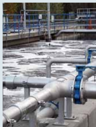
Air (O 2 ) – aeration of activated sludge basins (wastewater treatment plants)
