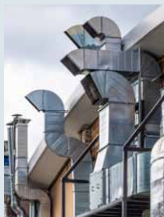
Air – fresh air in ventilation ducts
