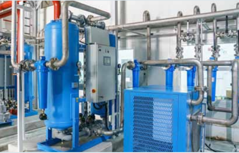
Compressed air – utilities
