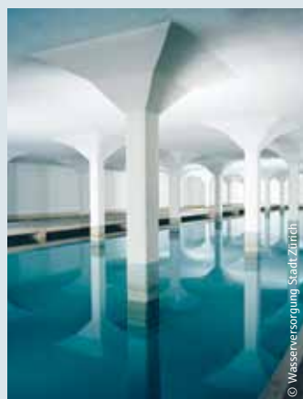
Ozone (O 3 ), chlorine (Cl 2 ) – disinfection of water
