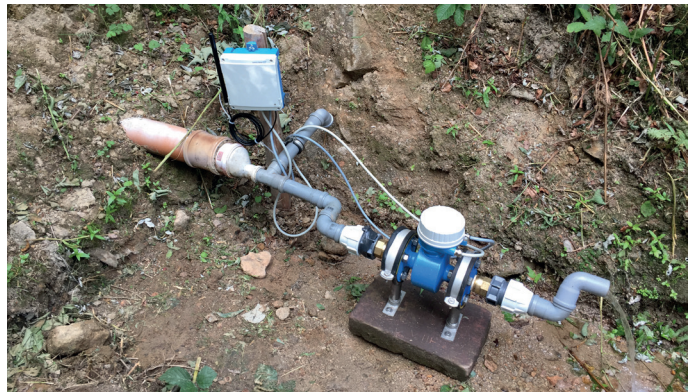
Measurement of a spring discharge with battery-powered Promag W 800
