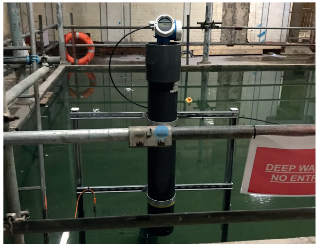
FMR60 radar installed in a stilling tube to eliminate outside influences
