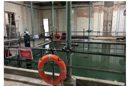
Monitoring the pool level
