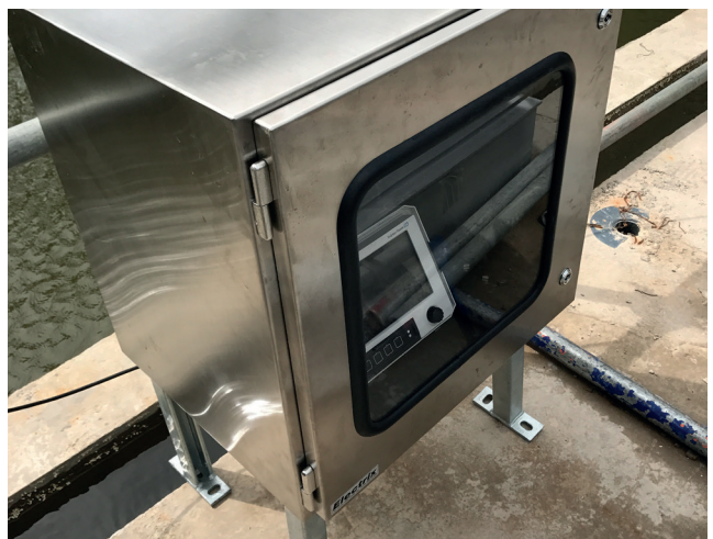
RSG45 data logger recording pool levels and temperature
