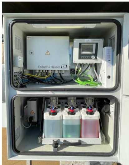
Main components in the transfer cabinet: CDC90 and pneumatic control unit as well as cleaning agents and pH buffer solutions
