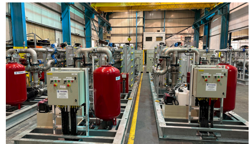
Torishima's cooling water systems
