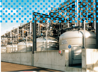
Caustic tank storage
