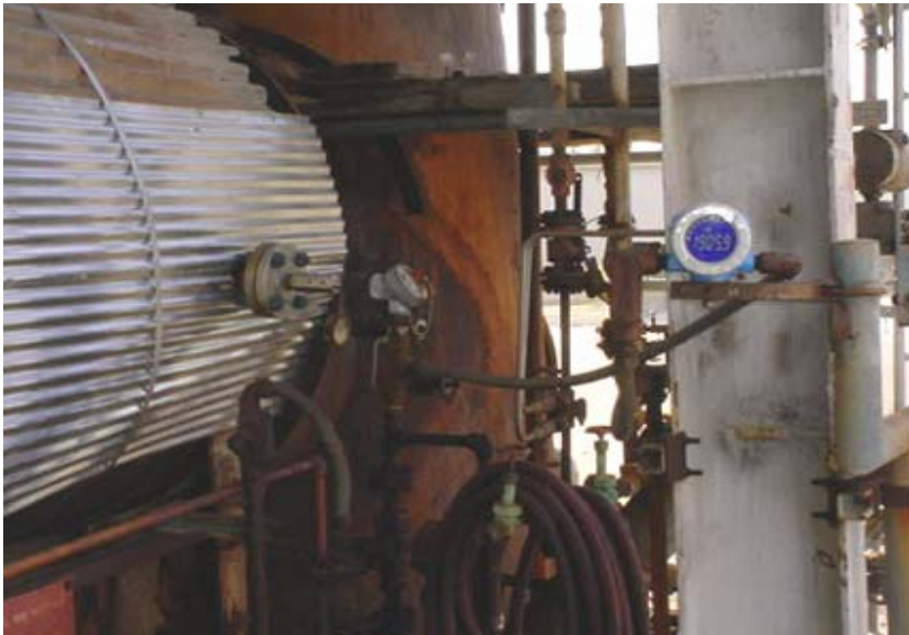
Temperature system installed in incinerator
