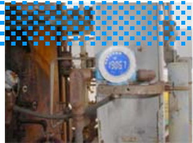
TMT 162 mounted outside incinerator
