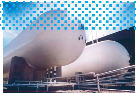
Steel storage tanks
